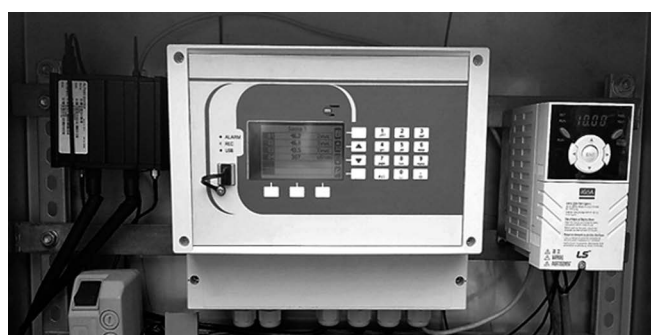
Figure 2. MPI-DN multichannel electronic recorder (middle) network connection router (left) and wave modulator for irrigation system (right) at research field in Nędza nursery farm (photo. G. Durło)
